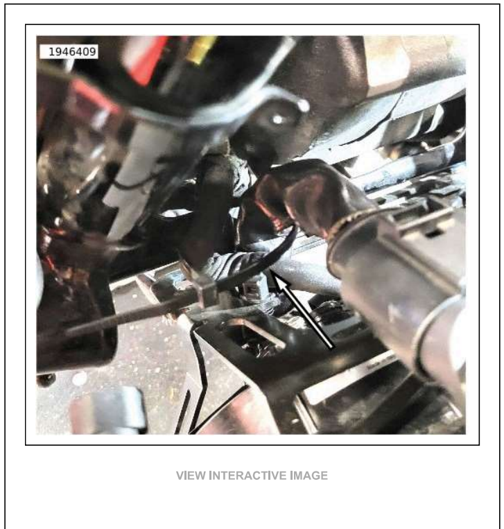
Figure 26. Loose Cable Strap
